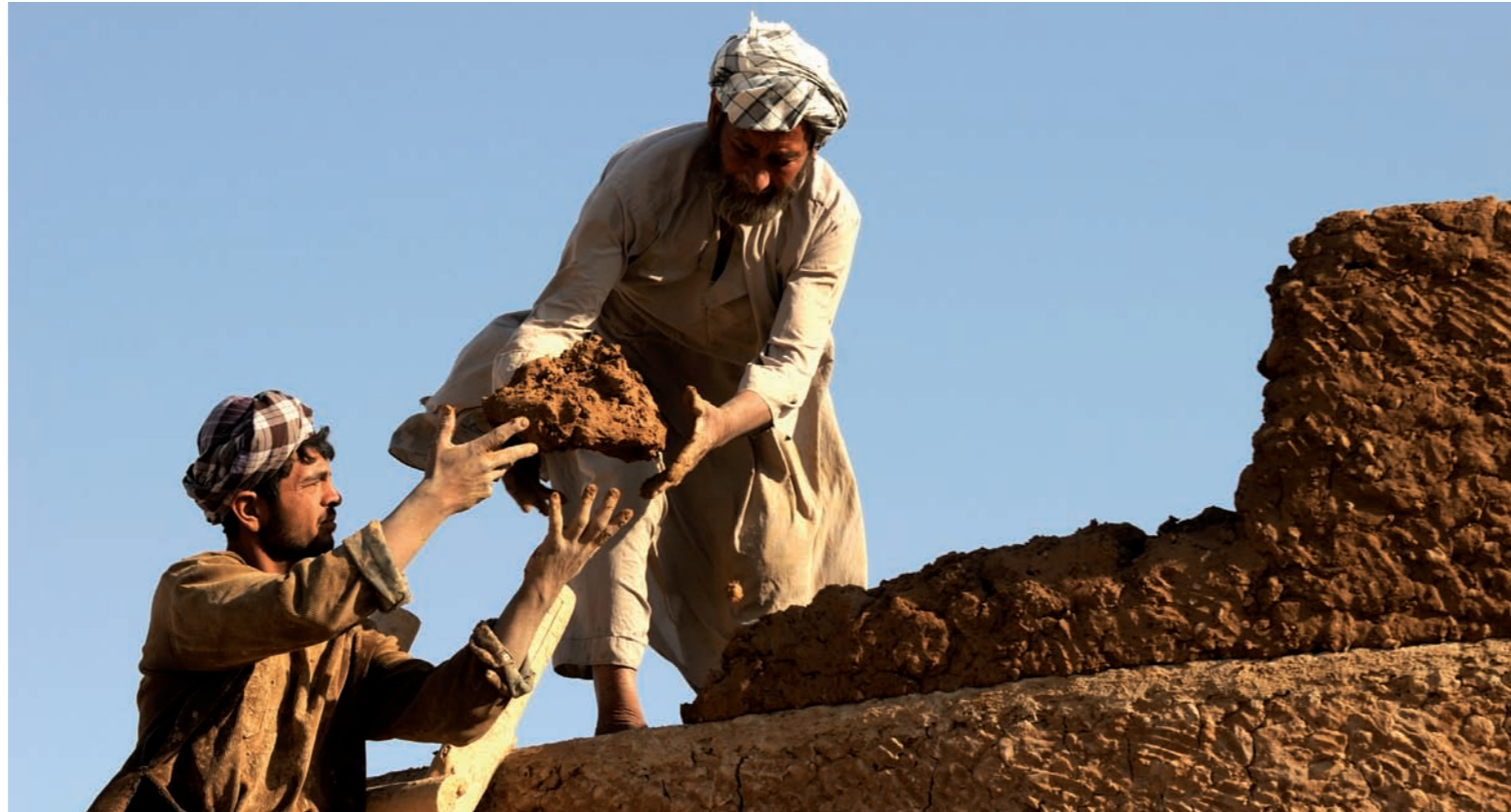
Making a new pakhsa layer on the garden wall of the Bagh-e Jehan Nama Palace.
