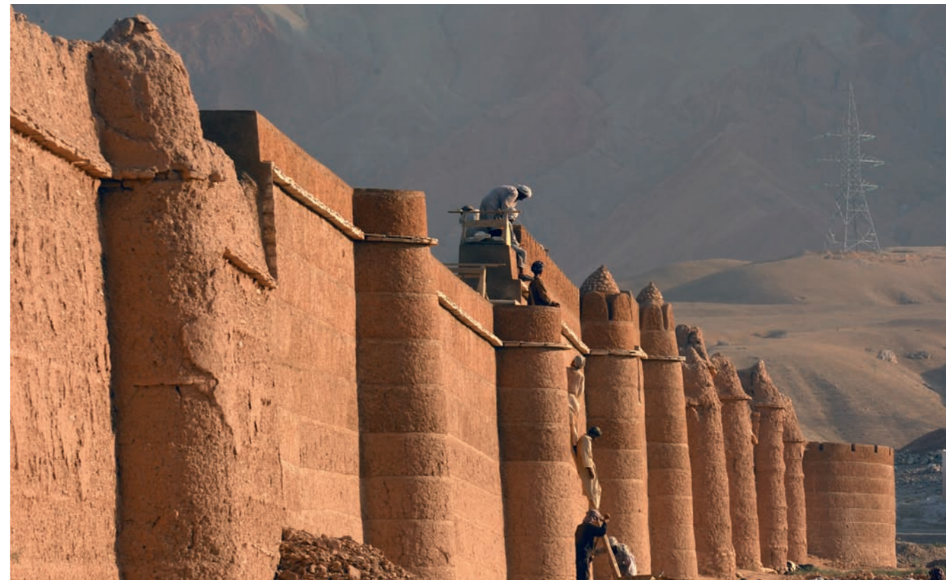
Building activities with the traditional pakhsa system at the palace garden wall of the Bagh-e Jehan Nama Palace.
